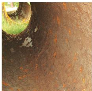
Figure 1: corrosion inside a cast iron pipe after 110 years (Gonzalez & Encalada, 2010)
